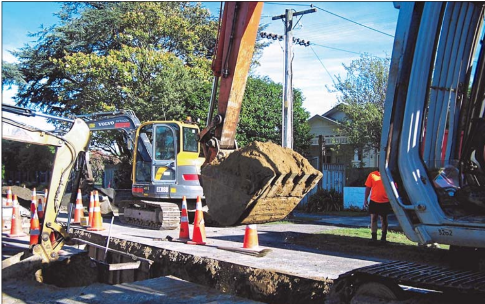
WORK is on schedule as contractors replace the sewer main and laterals (property connections) in Poole Street, Feilding, from East Street to Drake Street. Settled weather conditions have enabled Infracon Taranua to make steady progress and a new water main and laterals are also expected to be laid over the next week or two. Similar work is to be carried out in Nelson Street and is expected to start shortly.
