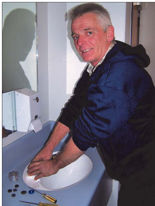
FEILDING plumber Trevor Hendra will soon be repairing a leaking cold water tap washer near you.
