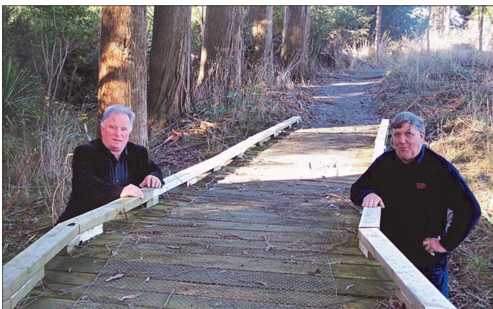
PARKS and Reserves Manager, Albert James (left), and Senior Community Work Supervisor, Barry Watson, inspect one of the bridges on the Mt Lees loop track.
